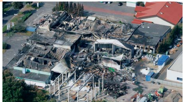
An impressive example of the properties of aerated concrete is provided by a fire that broke out on 31 August 2005 in a German paint factory. Here a technical defect in a warehouse for paints, varnishes and tanks of chemicals triggered a fire that spread not only to the production buildings of the paint factory but also to the production hall of an adjacent textile company. The extinguishing work was delayed by the explosion of several tanks of chemicals and was additionally greatly hindered by components flying around and the development of smoke. The result: the warehouse was completely destroyed and the production hall of the paint factory was almost completely destroyed. Only the hazardous goods store and the walls of the administration building were spared. Both of these were made from aerated concrete.
