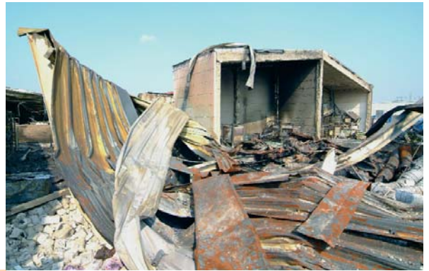
Typical image: After a large fire, a hall made from aerated concrete rises almost unscathed from the rubble. The rest of the factory was completely destroyed by the flames.
